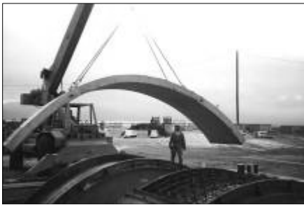
Precast panels are stripped from the forms daily and stored until sufficient concrete strength is reached
